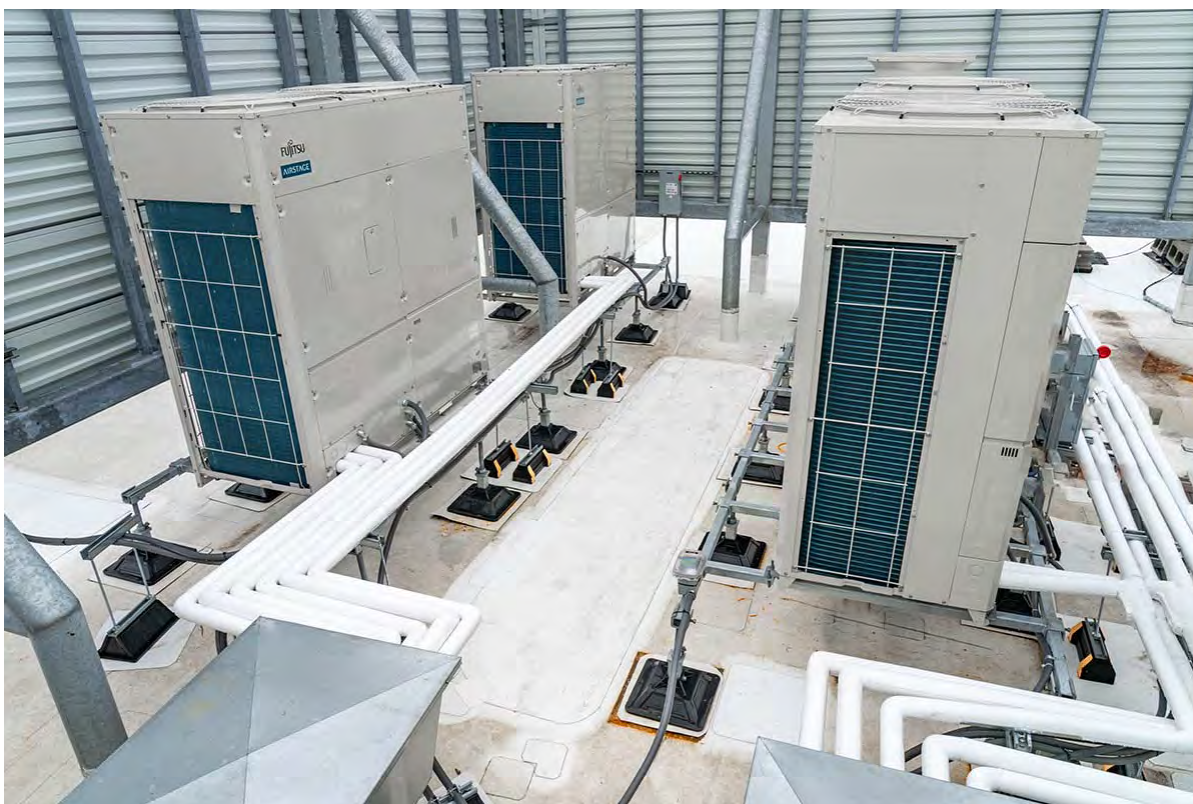
THREE PIPES: Observers can tell this is a heat recovery VRF system, as it has three pipes connected to the condenser, as opposed to two for heat pump systems. (Courtesy of Fujitsu AIRSTAGE)
