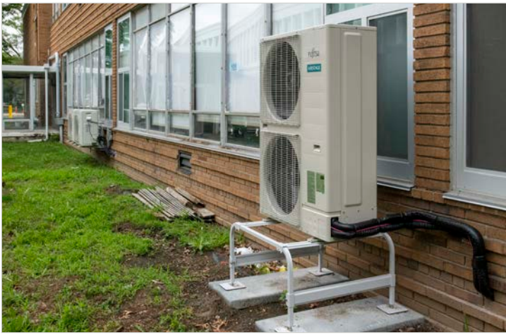
One of the school's four, five-ton AIRSTAGE J-IV condensing units mounted on a snow stand.
