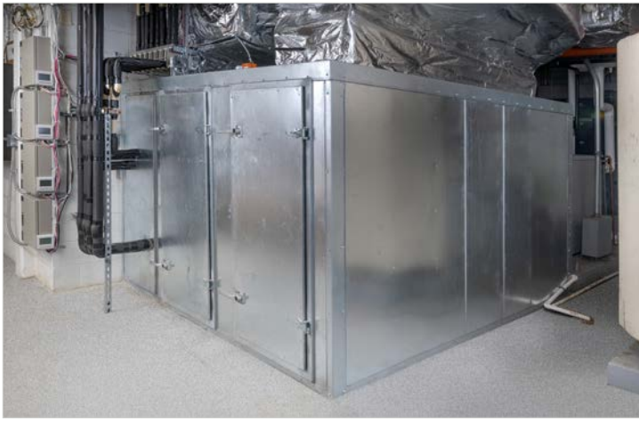
The retrofitted coil box containing a filter bank and the new coil.
